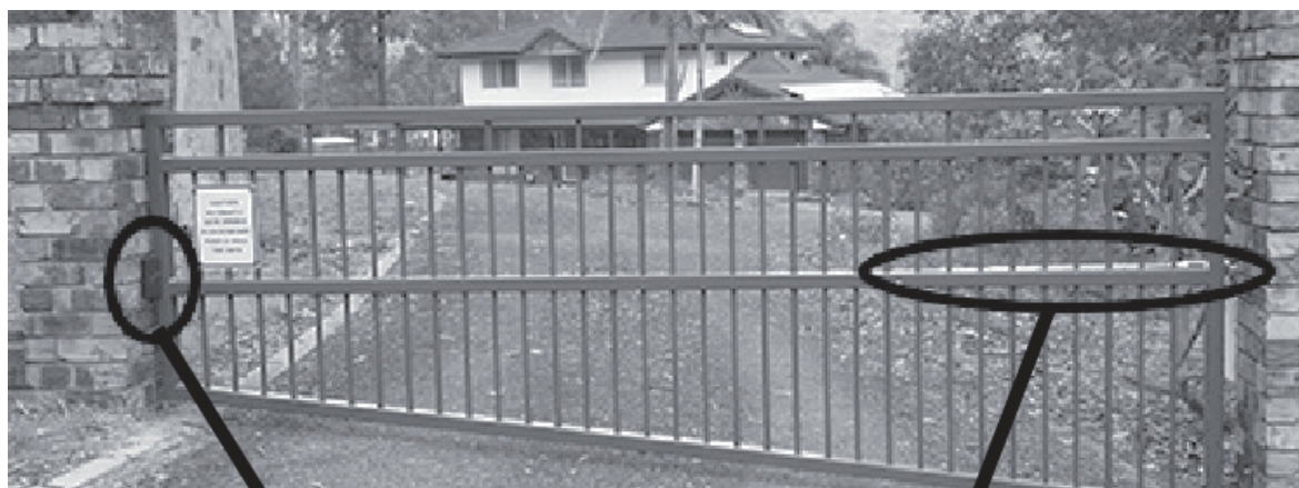
Rubber gate Stop on post
