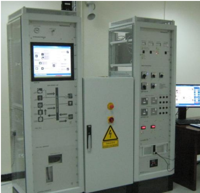
Fuel Cell System, Power Electronics, Energy Management
